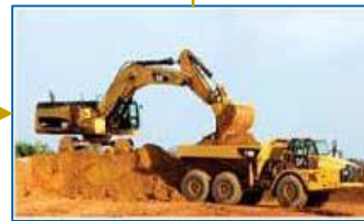
Conventional earth moving equipment to supply ore to the dry mining concentrator
