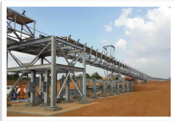
Oversize Conveyor Drive Area
