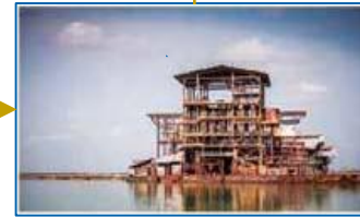
Wet plant to process the Dredge feed into a heavy mineral concentrate
