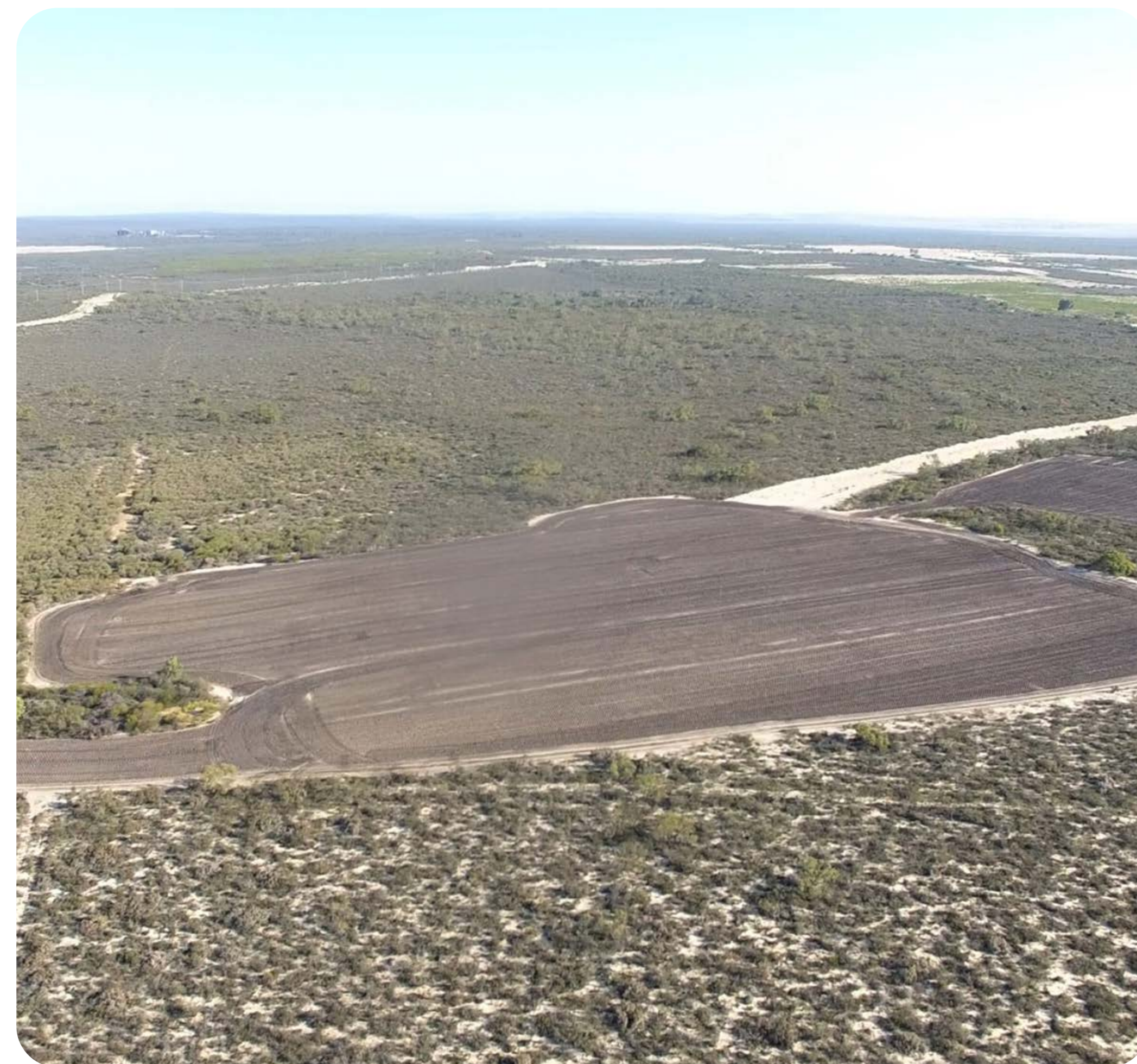
Completed native vegetation seeding of an old mining area and haul road
