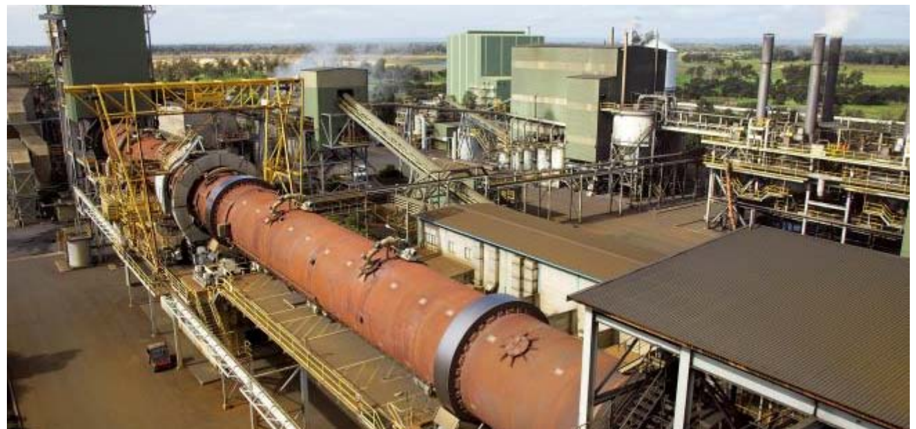
Synthetic rutile kiln in operation, Capel Western Australia
