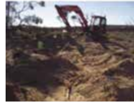
Excavating Western Myall surface and lateral roots – part of the initial scientific investigation with the University of Adelaide and Adelaide Botanic Gardens.
