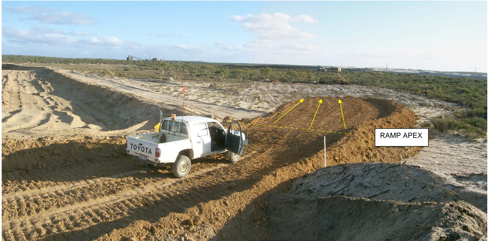
Hygiene ramp constructed with oversize material. Ramp section steps up immediately in front of LV with wash water returning to dieback infested area (vegetation in background)
